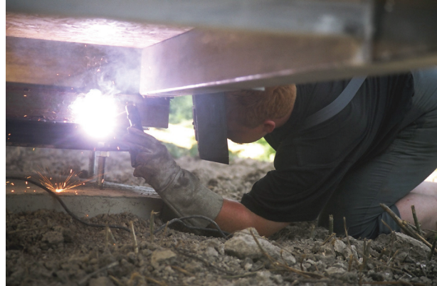
Figure 7: ... and welded onto the turntable, which had been put into an exactly horizontal position.
